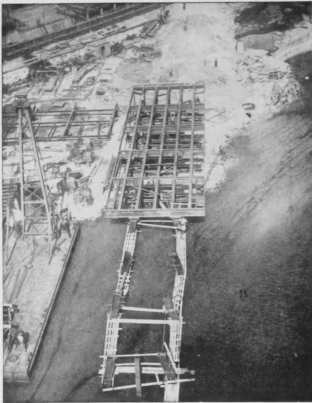
The new No. 1 (East) Finger Pier, now under construction, will be one of the largest all-welded steel oil-handling piers in the world. It will reach 790 feet from tip to shore, and will berth two 26,000 ton ocean tankers.
